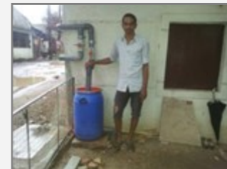
Rain Water Harvesting
